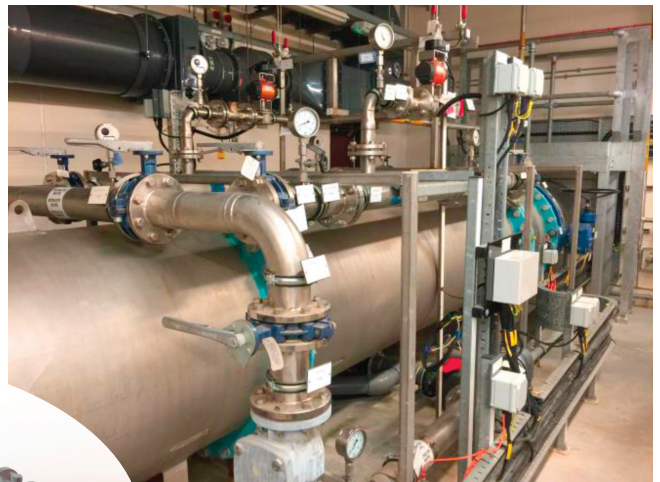
GDS installed at customer site
